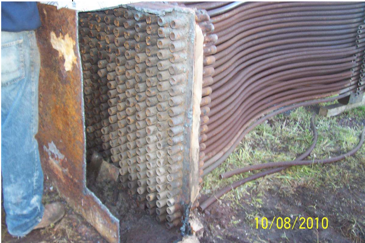
The bottom of the recuperator where the air passed from the carbon steel to the stainless steel rods.
