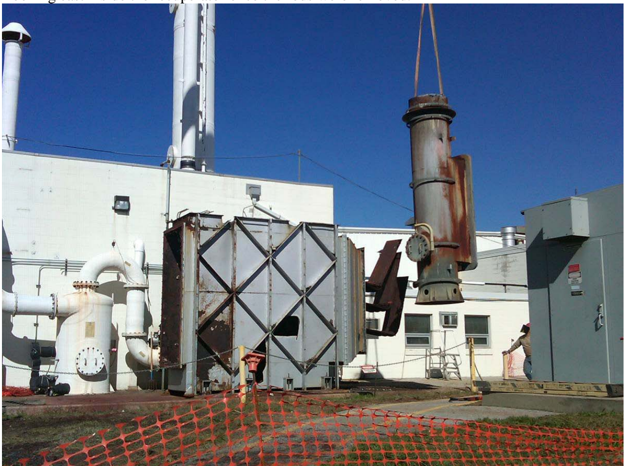
View of the east stack of the TFO (effluent side) being lifted off.
