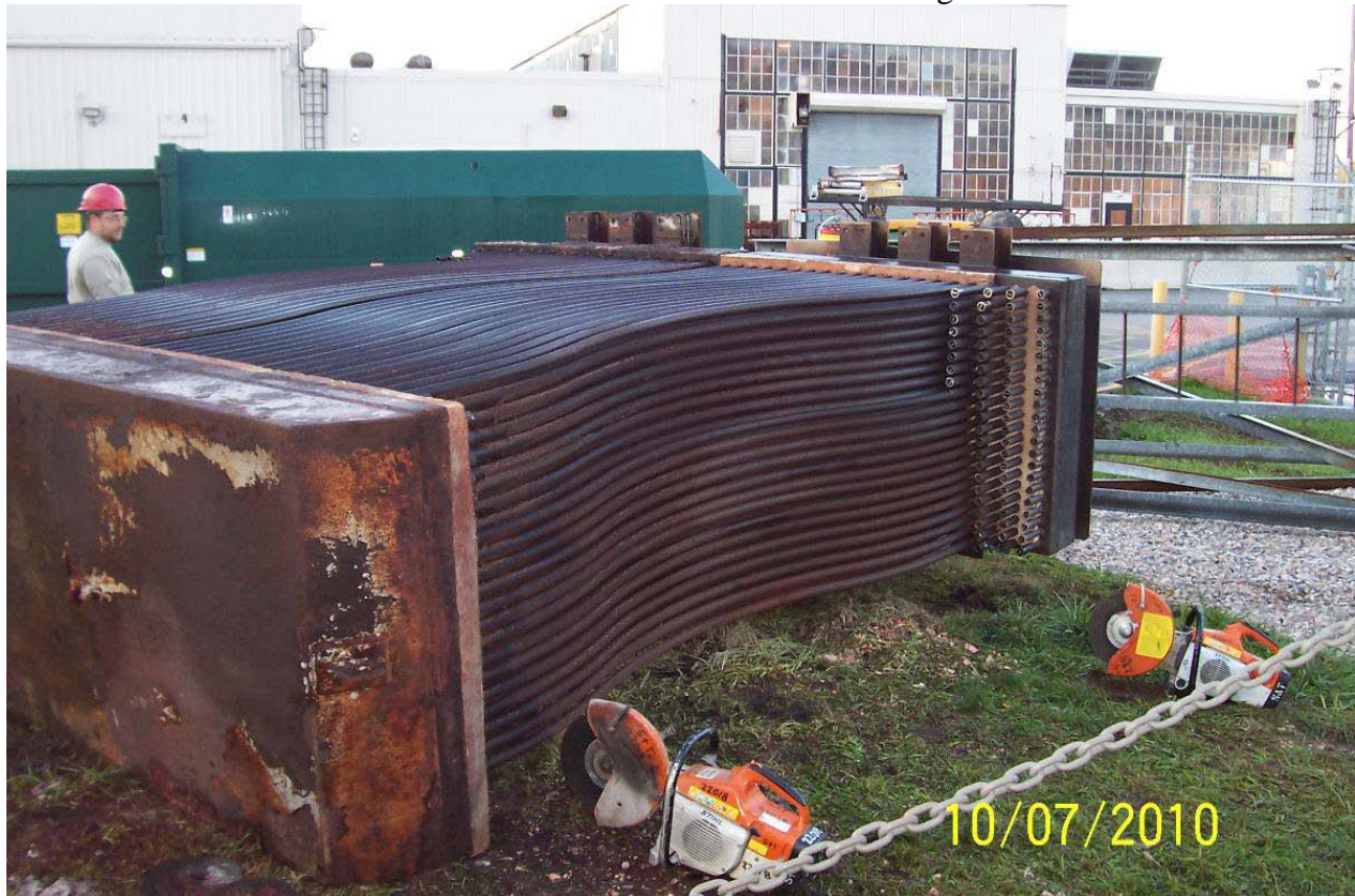
TFO recuperator rods are being removed for scrap. The near side is carbon steel and the far side is stainless steel. These corroded rods restricted air flow through the TFO.
