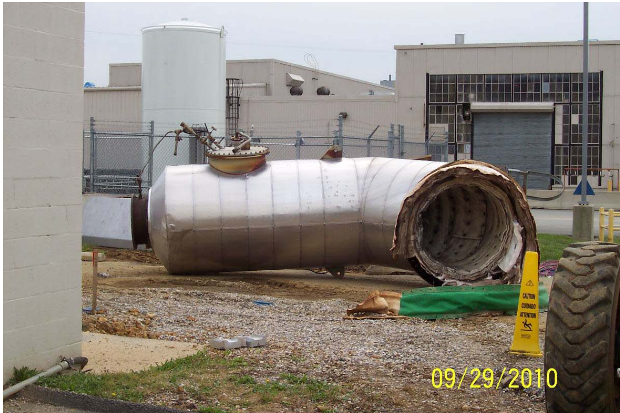
TFO burner on left side of stack and insulation can be seen on the right side of the stack.
